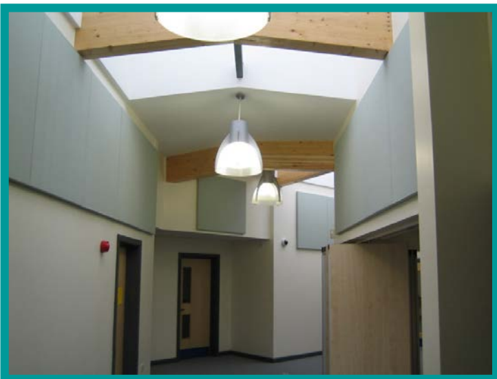
A hallway fitted with acoustic sound absorption panels
